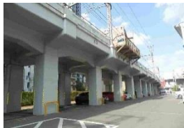
Elevated track pillars (Flexural failure type)
