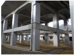
Elevated track pillars (Shear failure type)
