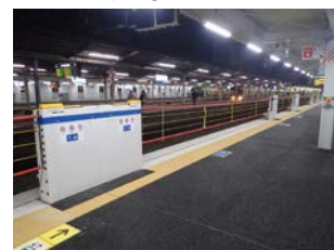
Automatic platform gates at Takatsuki Station
